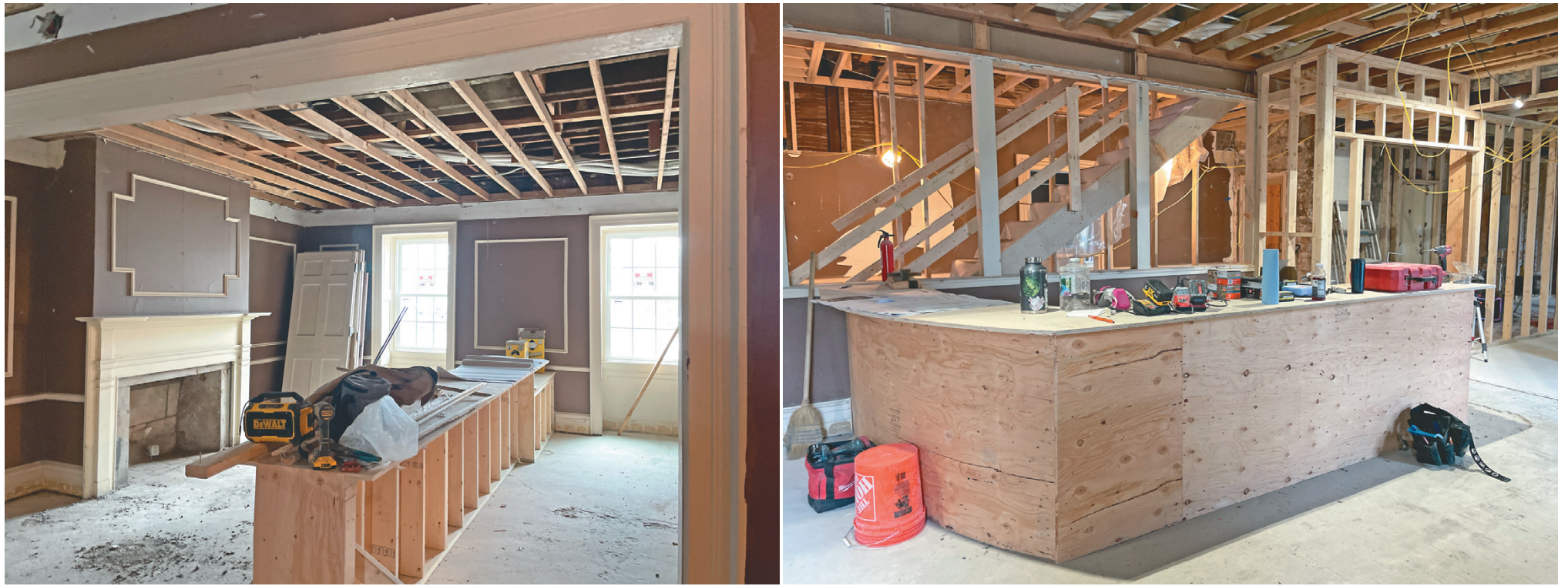
A look inside the Frontier House, as renovations continue toward a planned summer reopening. Clockwise: A first-floor side room. • A future Fairbanks restaurant bar. • An historic fireplace. • Upper-level metal framing. • The first-floor staircase. See more photos online at www.wnypapers.com.
